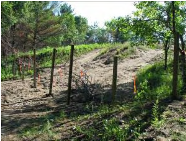
Fence built on the Barr Property in the Rice Lake Plains Natural Area to keep unauthorized ATV users from damaging the sensitive sand ecosystem. Photo: Todd Farrell
